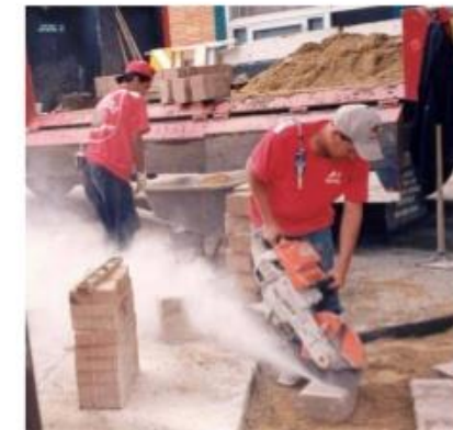
Without dust controls, using a handheld power saw to cut concrete can expose workers to high levels of respirable crystalline silica.
