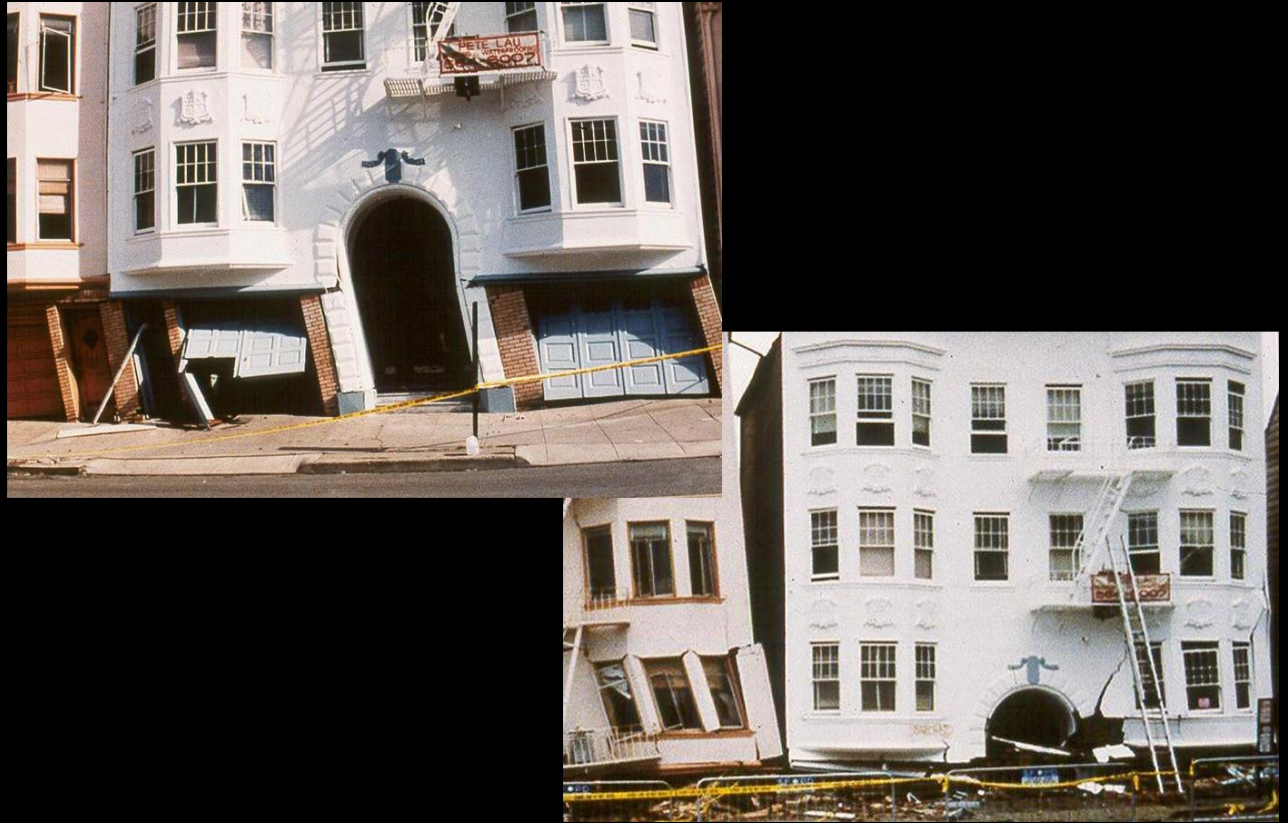
Loma Prieta Earthquake left building in hazardous condition
