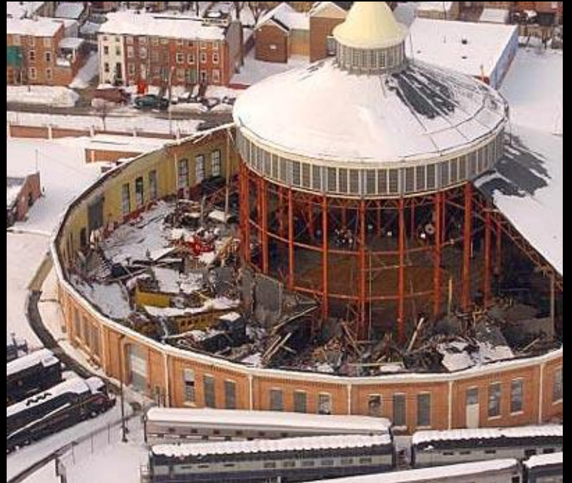
B&O Roundhouse Museum Collapse
